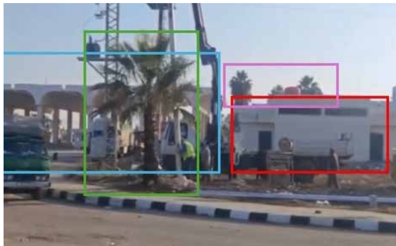
Figure 6: A screenshot from a video taken of repairs at the Nasib Border Crossing. Key features marked. Source: Facebook user @Khaled Iskef
